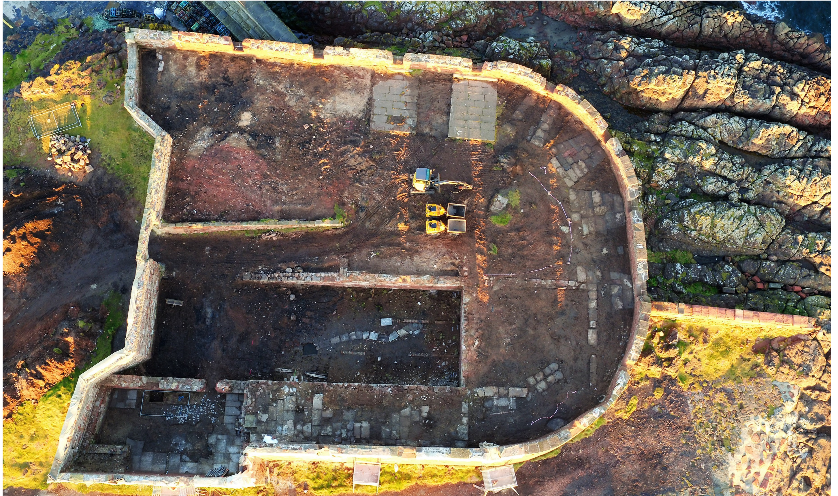
FIG. 13 Drone photo of the site during construction. Photo courtesy of Alistair Clark.
