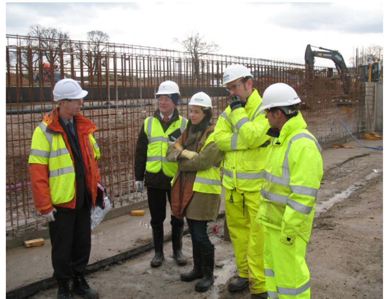
FIG. 21 Mackenzie with the design team on site. Photo courtesy of Graham Doig, Site Engineer.
