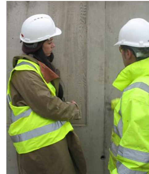
FIG. 20 Examining the concrete finish after the trial panels have been poured. Photo courtesy of Graham Doig, Site Engineer.
