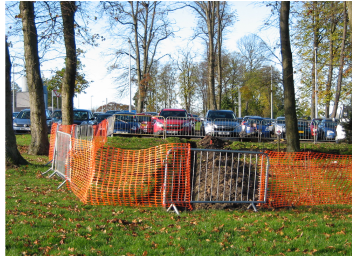
FIG. 7 Hand digging to locate tree roots prior to wall foundation design. Photo rankinfraser landscape architecture llp.
